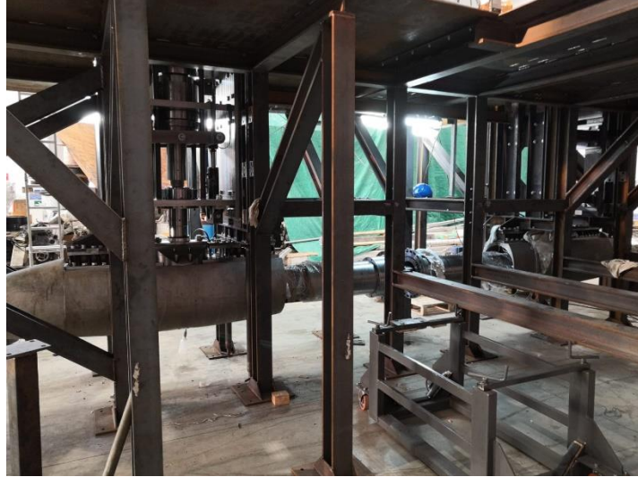
Figure 19. Installation phase of the two lower gearboxes and of the torque applying device in the test bench frame structure.
